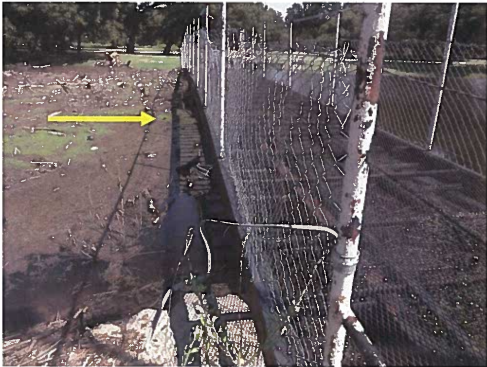
Photo No. 4: Lateral deflection of bridge observed (arrow depicts direction of debris impact)
