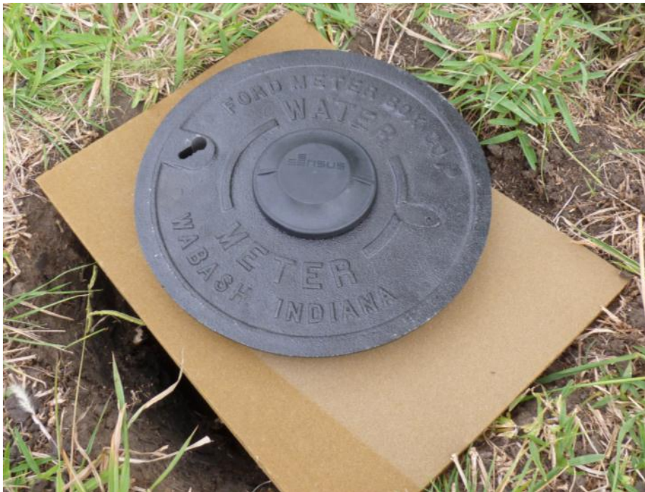
The Sensus water meter antenna is the small round bulge in the center of the cast iron pipe cover.
